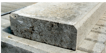
Stari beton, beton
